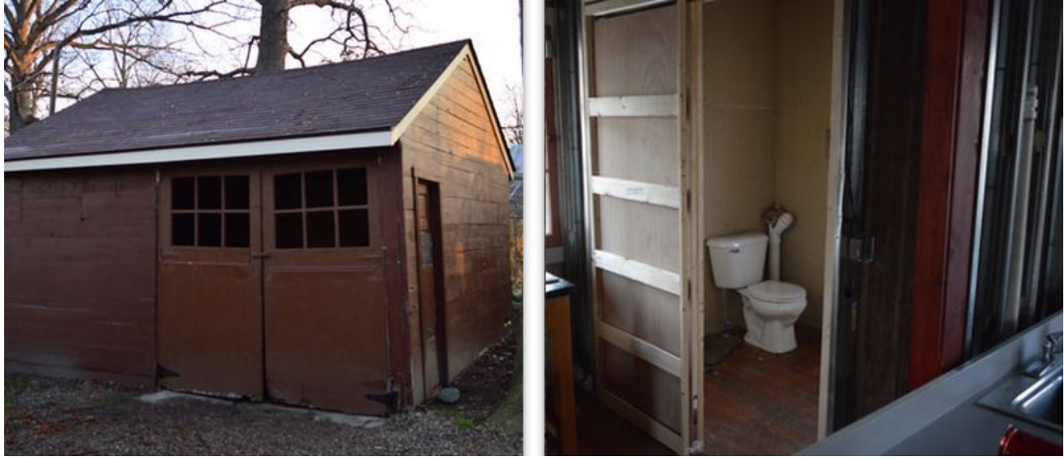
New shed roof pictured left, and bathroom frame and improvements on the right
